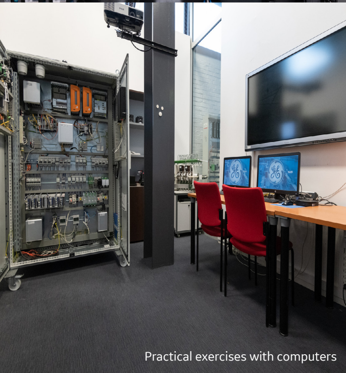
Low voltage components
